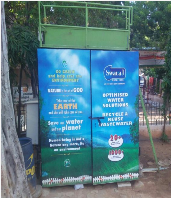
STP at Independence Day Park, Valluvar Kottam, Greater Chennai Corporation
