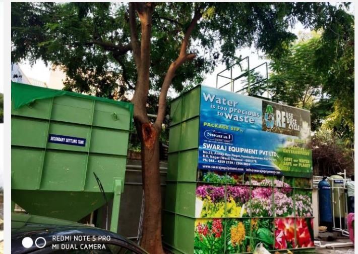
STP at 40 KLD at Aashiana Apartment, Chennai
