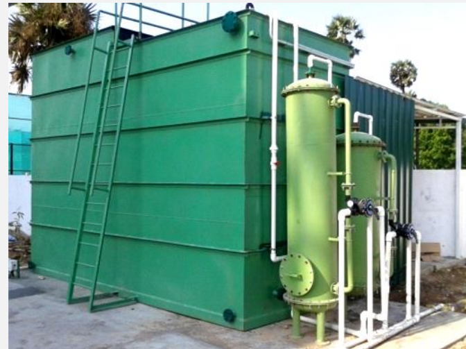
STP at 45 KLD at DRA, Pristine Pavilion, Mahindra City, Chennai
